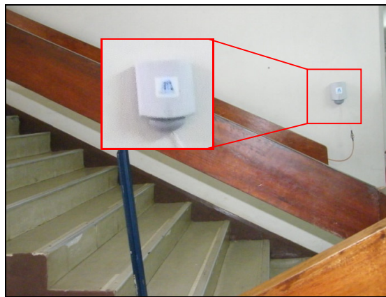
Figure 10. Plate Antenna placed at an entrance/exit point
